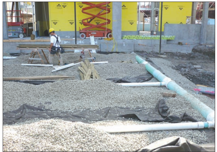
Perforated pipes divert stormwater into the rocky substrate beneath the parking lot's porous pavement, where it can be safely stored. Photo by Coughlin Porter Lundeen
